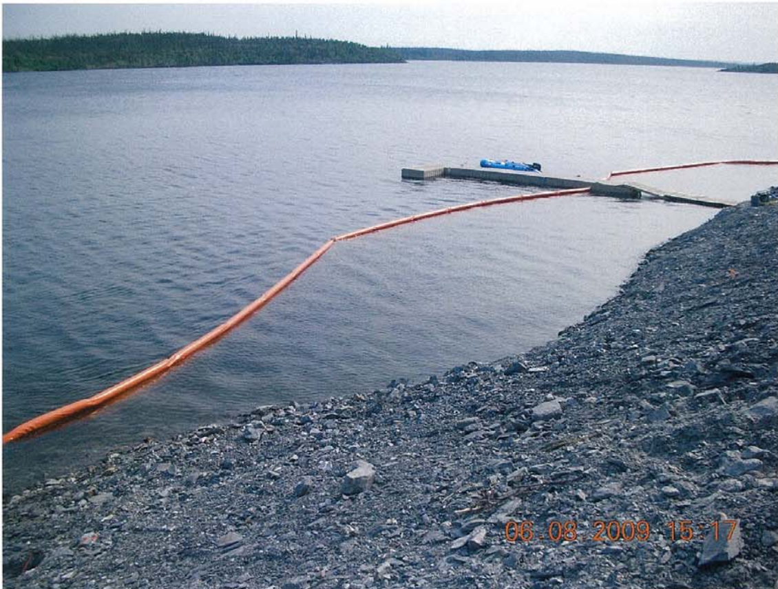
W2009X0002 - CARD - North Inca Remediation - Indin Lake, NT. Silt curtain deployed in Indin Lake prior to resloping the bank adjacent camp.
