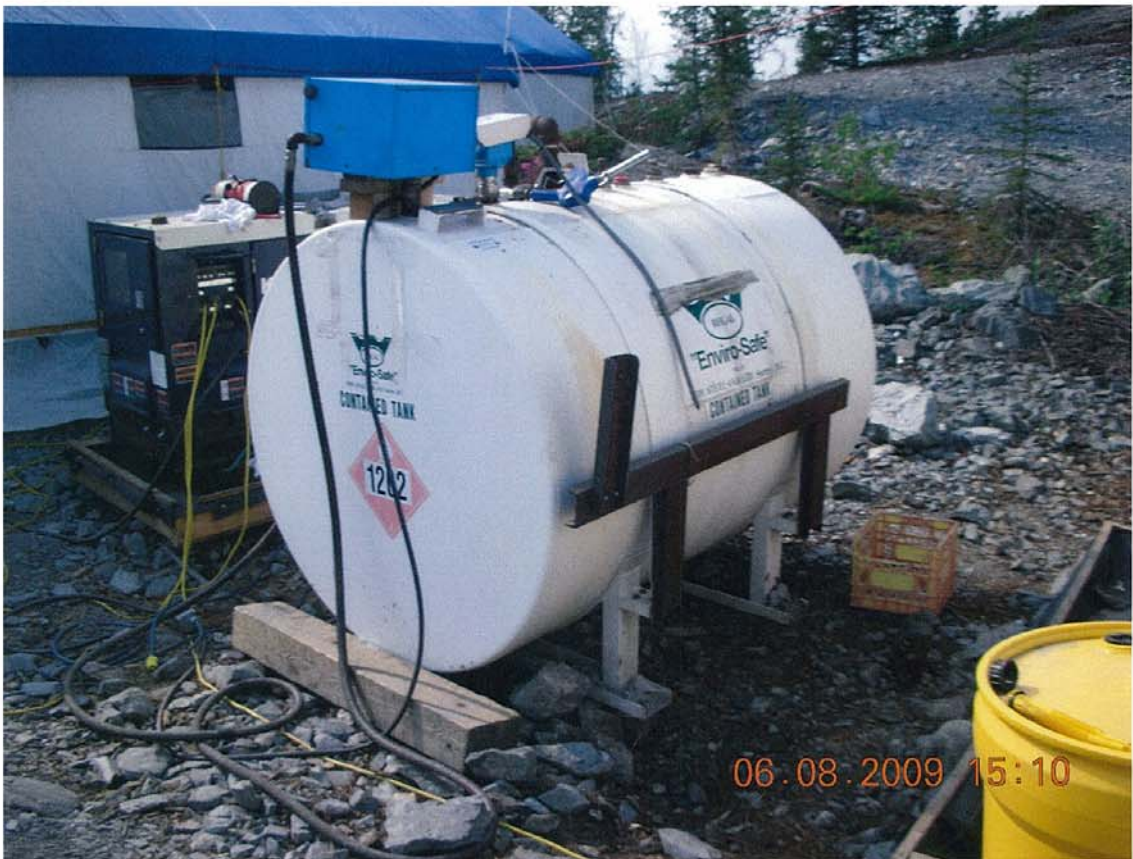
W2009X0002 - CARD - North Inca Remediation - Indin Lake, NT. Fuel storage within a 2500L enviro-tank and generator within secondary containment.
