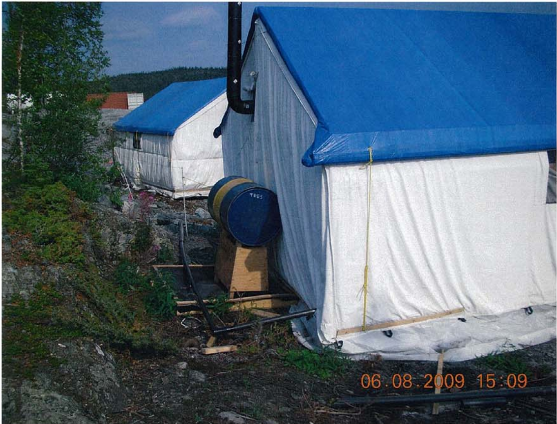
W2009X0002 - CARD - North Inca Remediation - Indin Lake, NT. All active drums have fittings wrapped with absorbents and are stored within secondary containment structures.
