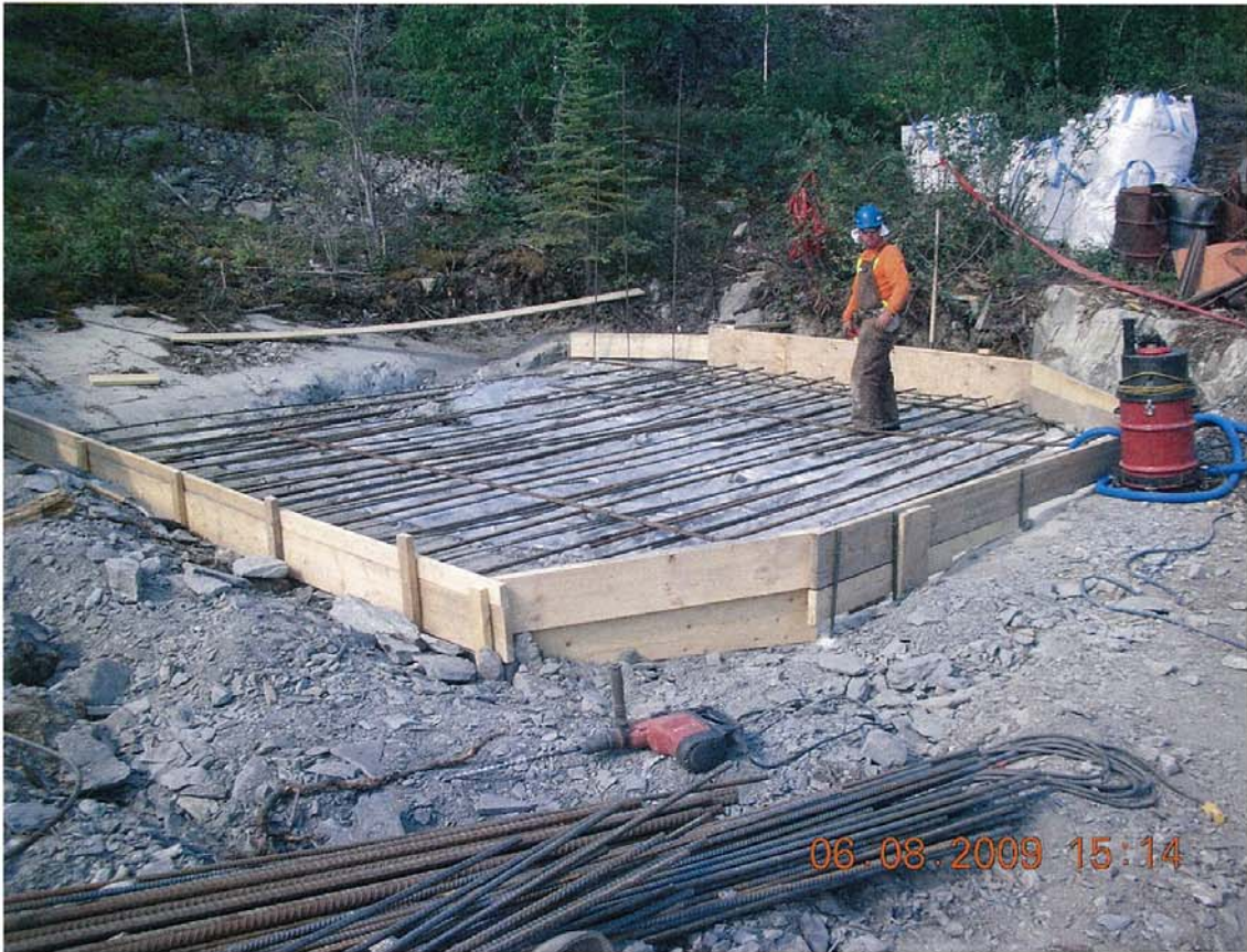
W2009X0002 - CARD - North Inca Remediation - Indin Lake, NT. Portal is being prepared for the installation of a concrete plug.
