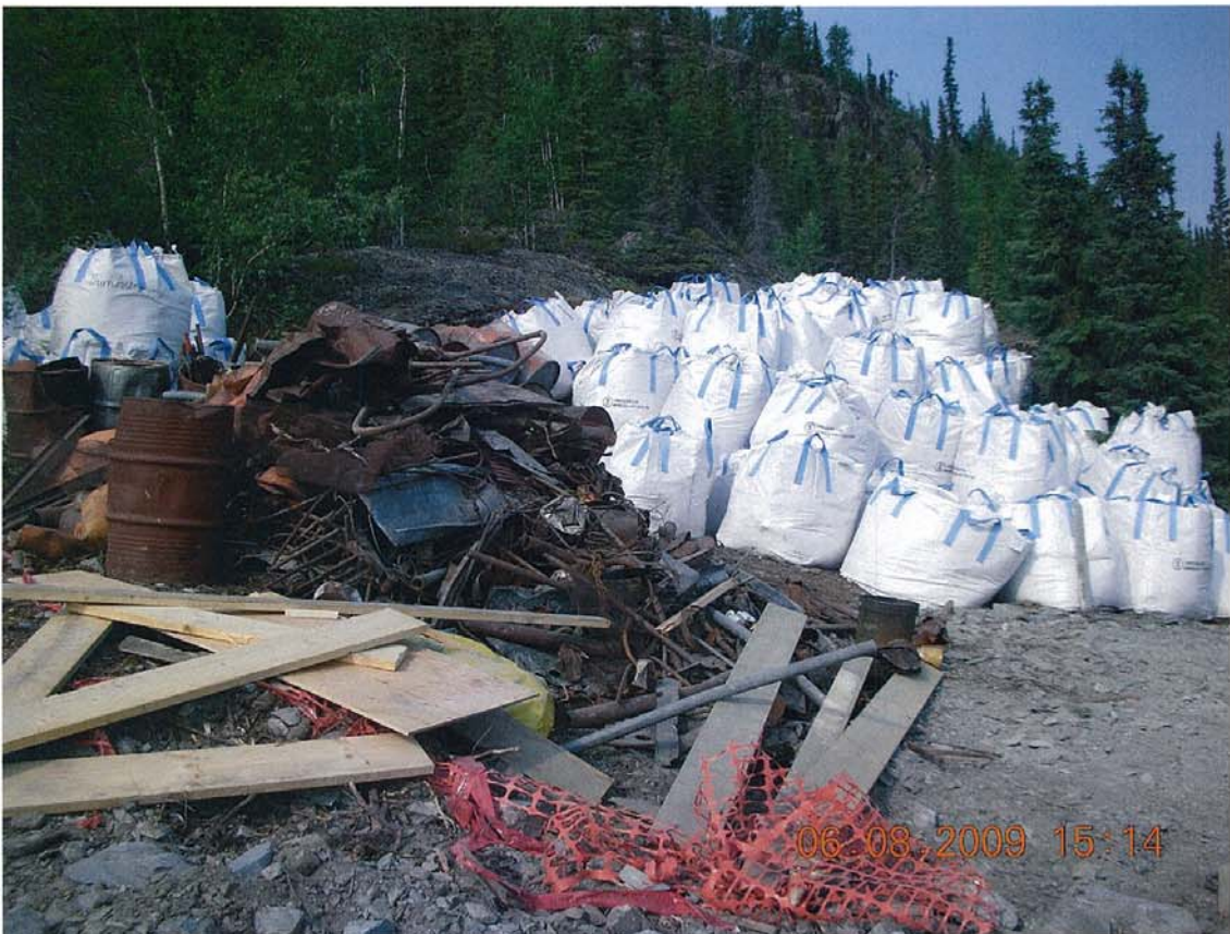
W2009X0002 - CARD - North Inca Remediaton - Indin Lake, NT. Waste metals and contaminated soils stored for back haul to Colomac for disposal in the landfill and landfarm.
