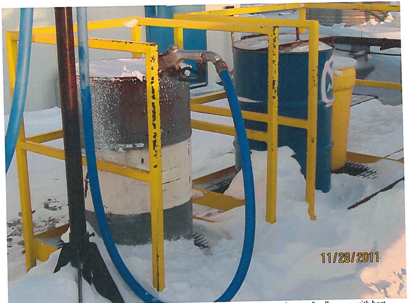
Figure 2. Effective fuel management at the fuel transfer facility (secondary containment & adherence with best practices).
