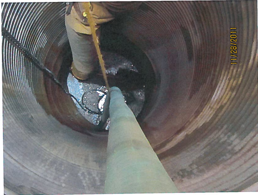
Figure 1. Seepage flows in the well at “EPKC Sump 1”. At the time of inspection, this water was being pumped back to the PKC Facility (as per Part H of the W.L.) at a rate of 1.5 L/sec (down from 4.5 L/s in mid October). The green hose (photo bottom) is the hose returning seepage water to the PKC. The large yellow duct (photo top) is directing hot air into the hole to keep the seepage water from freezing.
