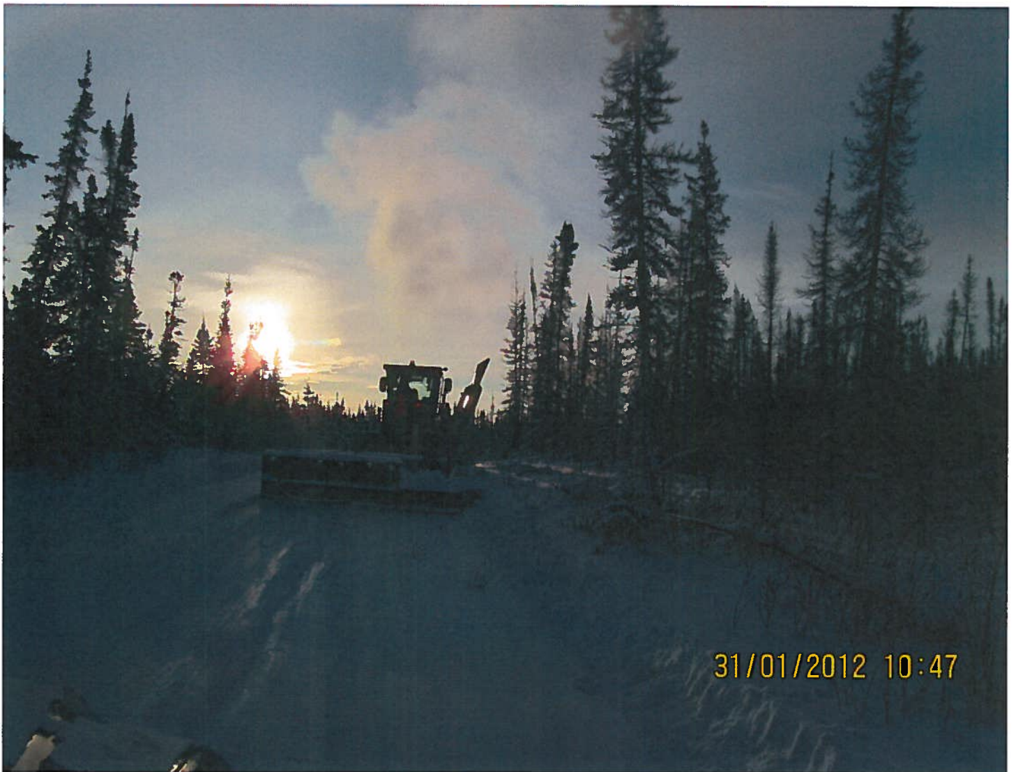
W2007F0001 - NTPC - Winter Road - Km 4 of the Wekweeti Road to Snare Forks. Photo #1 - Grader hauling drag along the winter road route.
