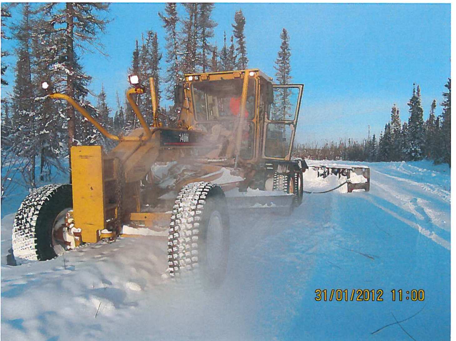
W2007F0001 - NTPC - Winter Road - Km 4 of the Wekweeti Road to Snare Forks. Photo #2 - Another photo of the grader and drag along the winter road route.
