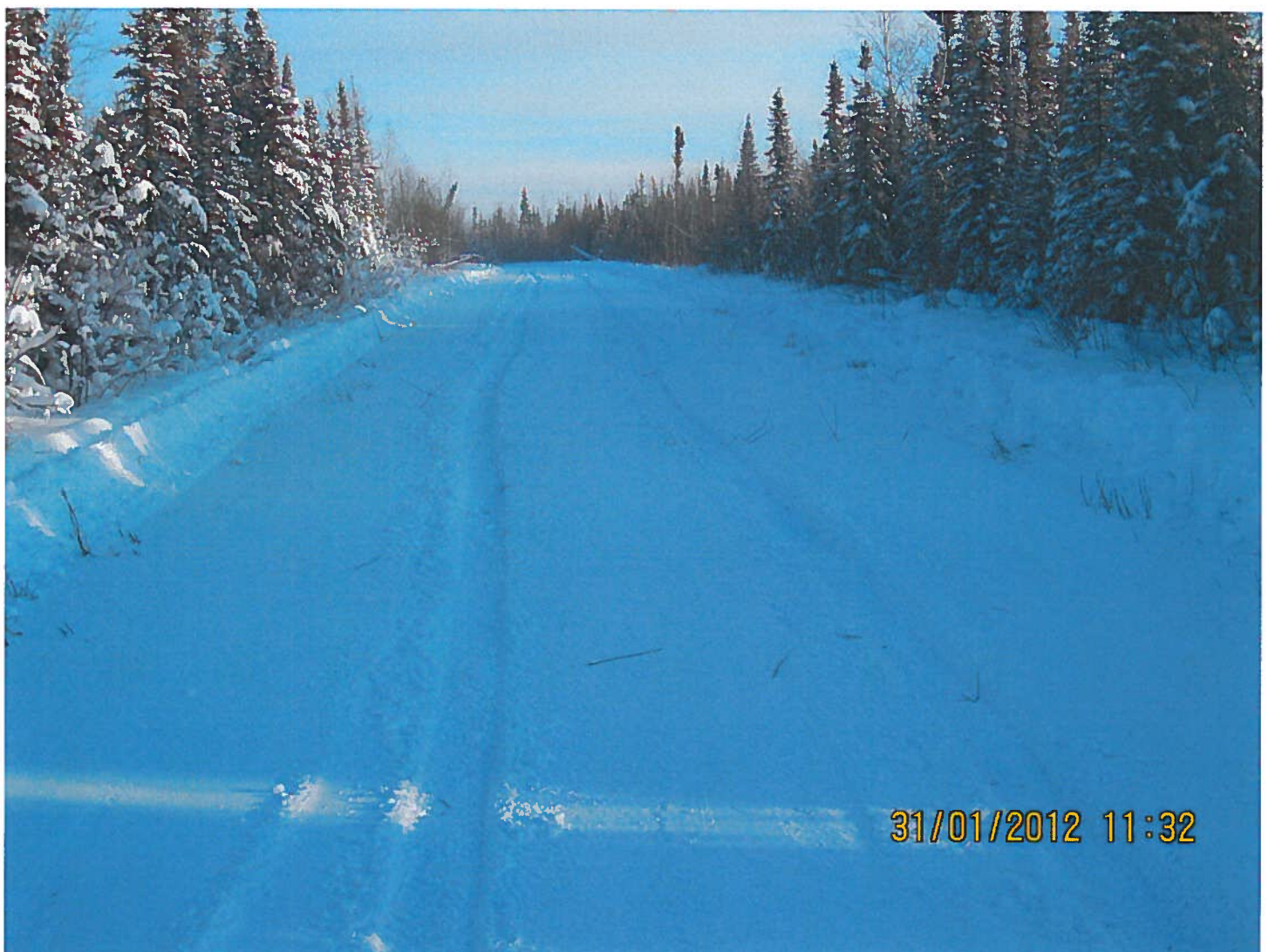
W2007F0001 - NTPC - Winter Road - Km 4 of the Wekweeti Road to Snare Forks. Photo #4 - More rutting from a pickup. Prior to hauling materials the road surface must be capable of supporting haul traffic.
